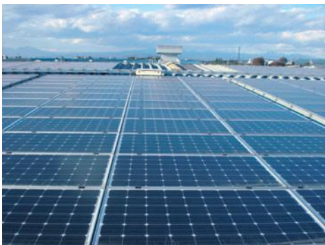
Photovoltaic power generation system on building owned by SMK subsidiary in Japan
