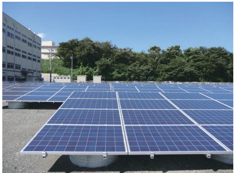
Kitaibaraki photovoltaic power plant at the Hitachi works
