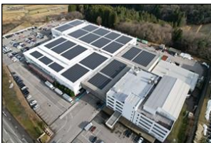
Solar power generation equipments (rooftop)
